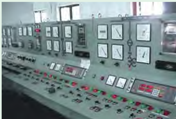
Automation of electricity production, transmission and distribution helps in the effective cost management
